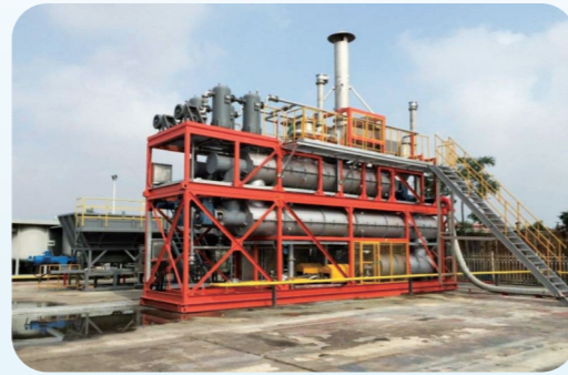
热脱附设施 Thermal desorption facility
