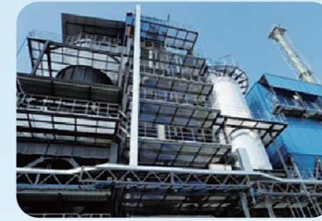
非焚烧处置技术 Medical waste non- incineration facilities
