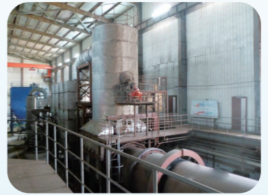
高浓度PCB回转炉焚烧处置设施 Rotary furnace incinerator for high concentration PCB
