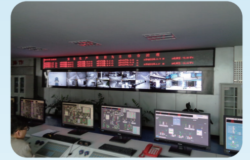
垃圾焚烧处置监控系统 Monitoring system for waste incineration and disposal
